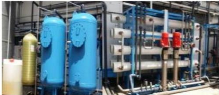
Reverse Osmosis water treatment systems
