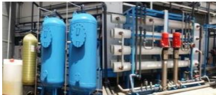
Reverse Osmosis water treatment systems
